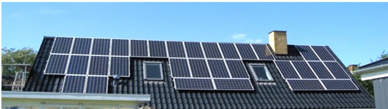
Chile 1.5KW Home On-grid System
